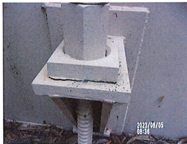
Showing gaps in the anchor chairs from the tank settling.
