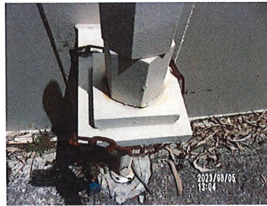
Showing rust stained from chains on the anchor chairs.
