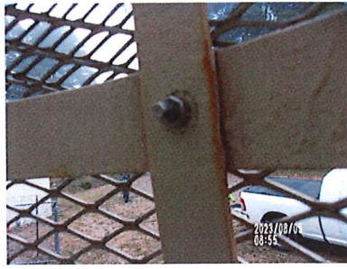
Rust bleed from inaccessible gaps.
