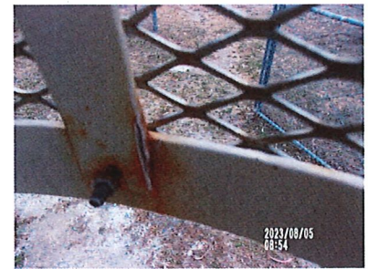
Example of ladder cage to be prepped caulked and re-coated.
