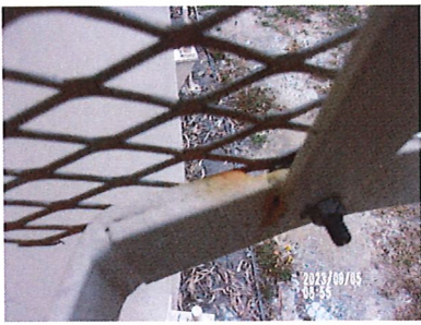
Ladder with rust bleed
