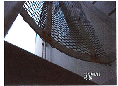
Isolated locations of the ladder cage to be touched up.
