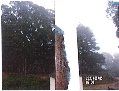
Showing what appears to be mil scale on the shop coated ladder cage.
