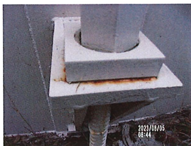
Rust leeching from the top of the anchor chair and bottom of the washer.
