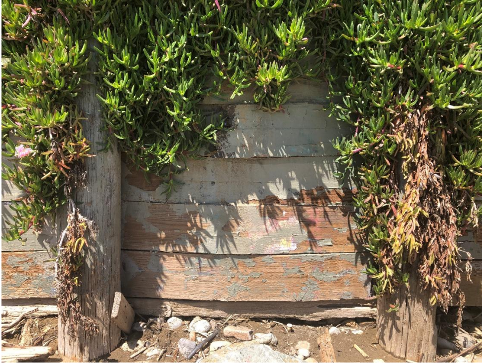
Photo 5: Severely bowing/failing timber lagging. Photo: IMG_3310.jpg Date: 4/13/23
