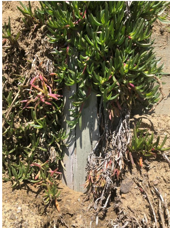
Photo 3: Vegetation growing from within void of split pile. Note sloughed slope debris around pile. Photo: IMG_3298.jpg Date: 4/13/23
