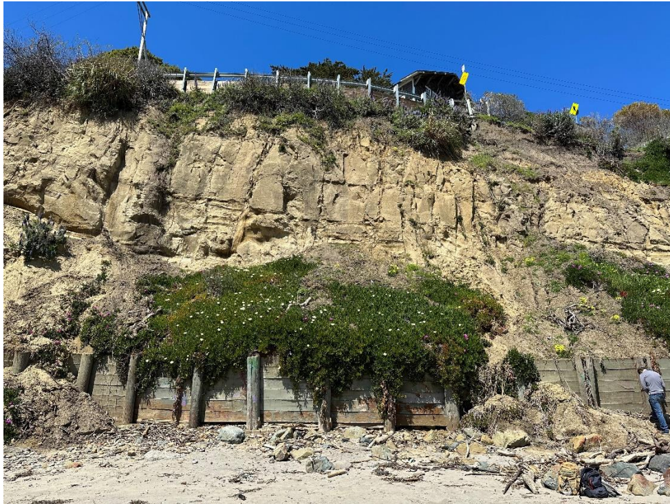
Photo 9: Sloughed material from upper bluff. Photo: IMG_0371.jpg Date: 4/13/23
