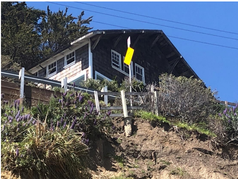
Photo 10: Undermined fence post on the upper bluff. Photo: IMG_0371.jpg Date: 4/13/23
