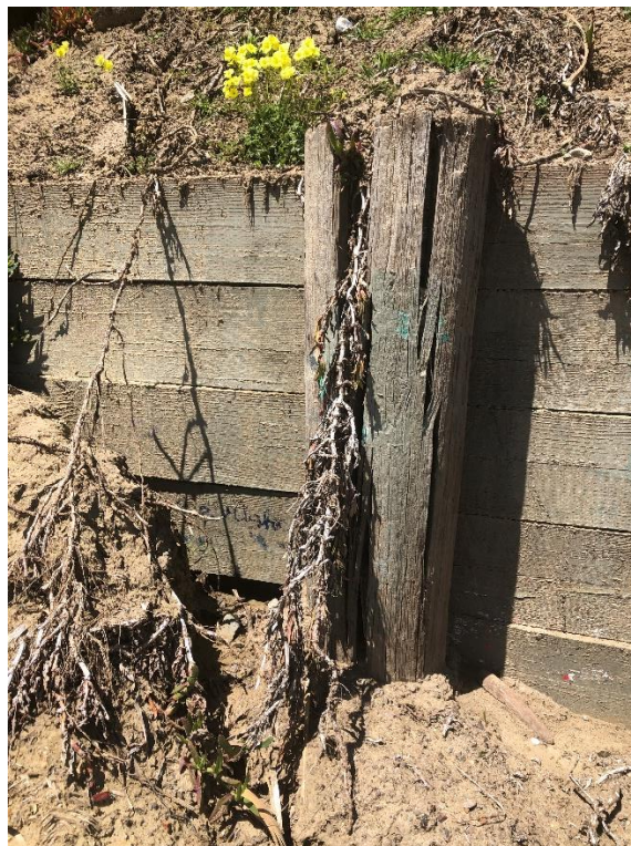
Photo 2: Debris and vegetation accumulation within void of split pile. Note missing bottom lagging at lower left. Photo: IMG_3297.jpg Date: 4/13/23
