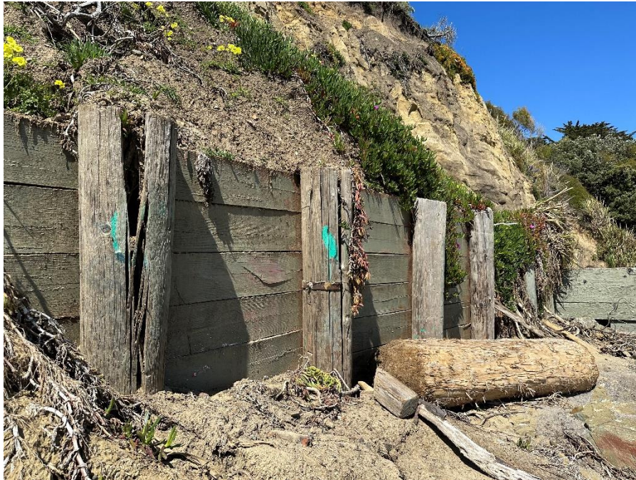
Photo 1: Severely split/failing sea wall piles. Note broken steel band at mid-height. Photo: IMG_3296.jpg Date: 4/13/23
