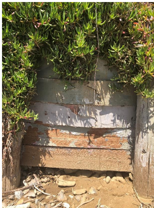
Photo 4: Severely bowing/failing timber lagging. Photo: IMG_3309.jpg Date: 4/13/23
