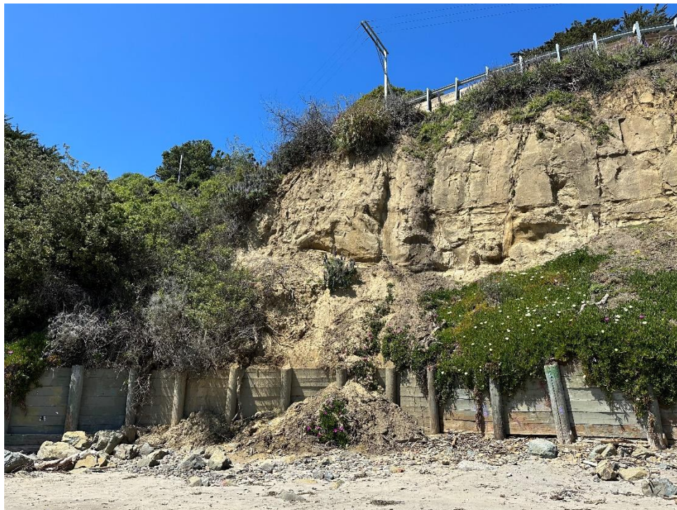
Photo 8: Sloughed material from upper bluff. Photo: IMG_0370.jpg Date: 4/13/23
