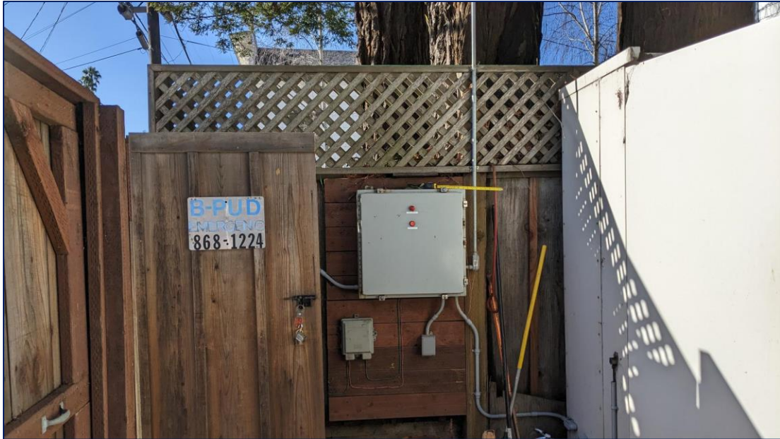
Existing Lift Station Autodialer Panel
