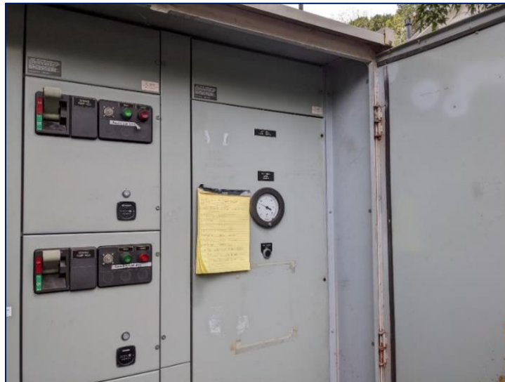
Existing Lift Station Motor Control Center
