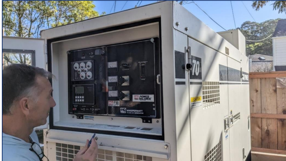
Existing Lift Station Portable Generator
