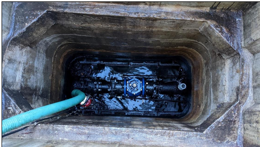
Lift Station Force Main in Wharf Road
