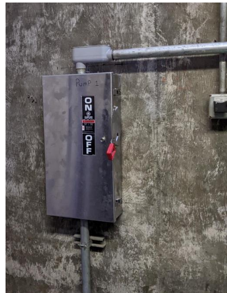
Existing Dry Well Pump Disconnect (Not Explosion Proof)
