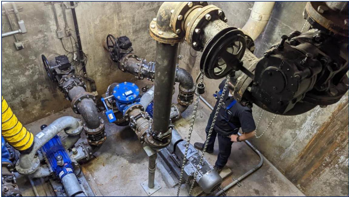
Existing Dry Well With Sewage Pumps
