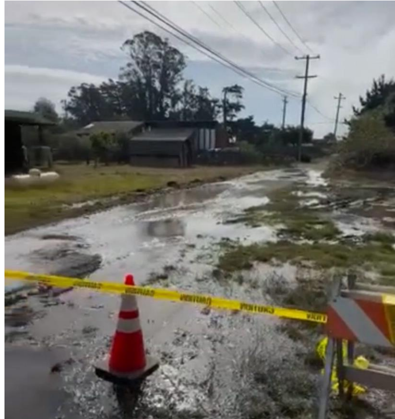
Large leak on Birch this past week
