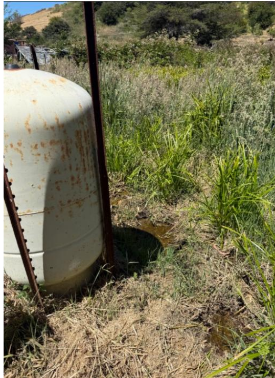
Resource Recovery Well
